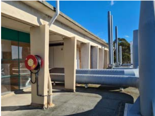
Building 17 - Chemistry, Central Science Laboratory Detail of the tapered rectangular columns on the rooftop Source: Paul Davies Pty Ltd
