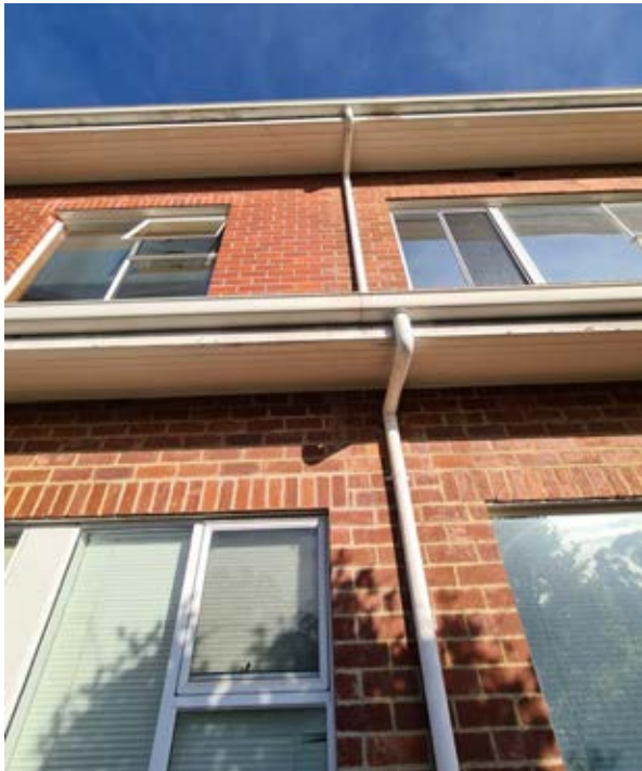
Building 38 – Research House Evidence of the first floor extension to the east can be seen in the change in brickwork on the first floor and evidence of the former mitred corner to the first floor eaves lining. Source: Paul Davies Pty Ltd
