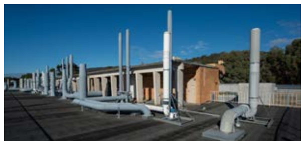
Building 17 - Chemistry, Central Science Laboratory View of the roof top Source: Paul Davies Pty Ltd
