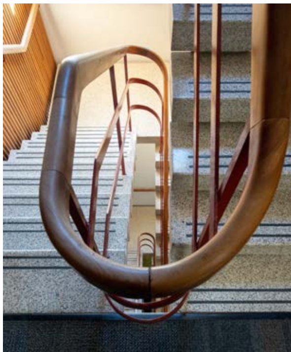
Building 26 – Psychology, Social Sciences Detail of the timber handrail Source: Paul Davies Pty Ltd
