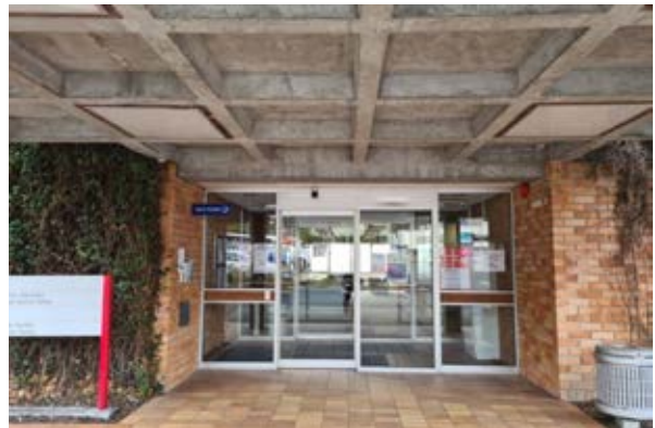
Building 29 – Humanities Building Detail of cast concrete ceiling to the entrance portico Source: Paul Davies Pty Ltd
