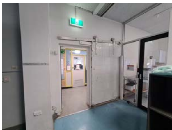
Building 17 - Chemistry, Central Science Laboratory Detail of original steel sliding fire doors Source: Paul Davies Pty Ltd
