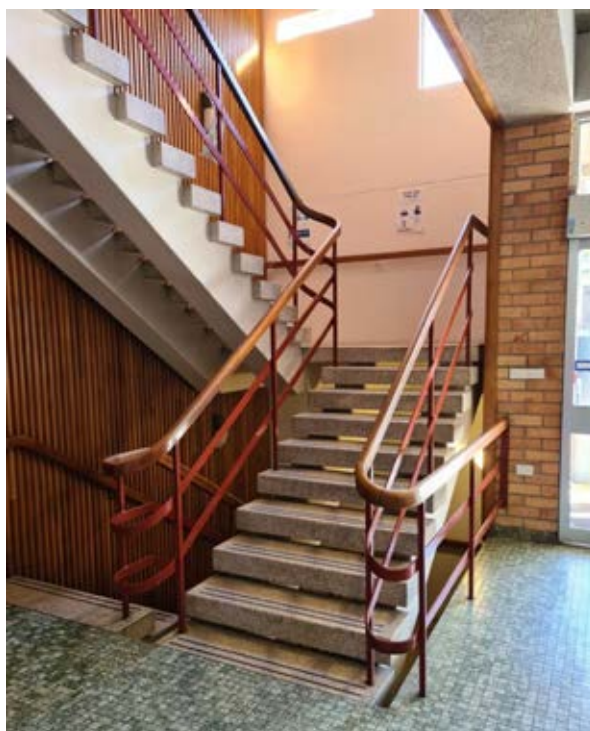
Building 26 – Psychology, Social Sciences Detail of the main entrance foyer stair Source: Paul Davies Pty Ltd
