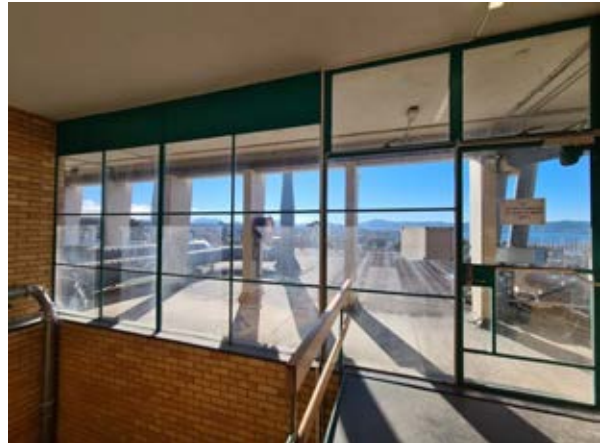
Building 17 - Chemistry, Central Science Laboratory View of the steel curtain glazing to the rooftop Source: Paul Davies Pty Ltd
