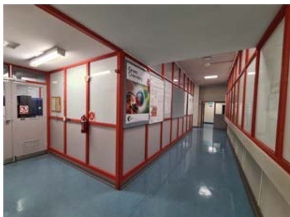
Building 17 - Chemistry, Central Science Laboratory Typical timber joinery to labs Source: Paul Davies Pty Ltd
