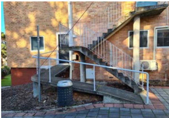
Building 21 – Tasmania University Union External stair and ramp to the northern wing Source: Paul Davies Pty Ltd
