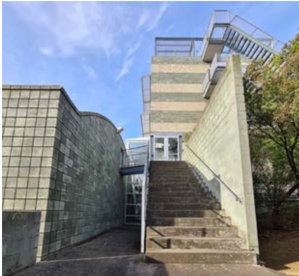
Building 40a –International Pathway College Western fire exit stairs Source: Paul Davies Pty Ltd
