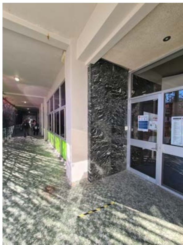
Building 26 – Psychology, Social Sciences Detail of the original green floor tiles and marbled wall panel adjacent to the main entrance Source: Paul Davies Pty Ltd
