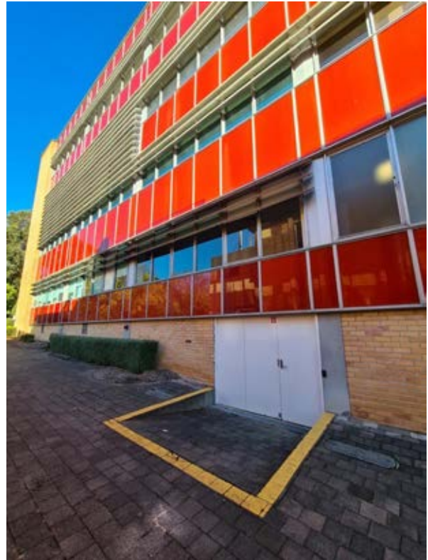
Building 23 – Library, Morris Miller Detail of the coloured glass curtain wall to the northern facade Source: Paul Davies Pty Ltd
