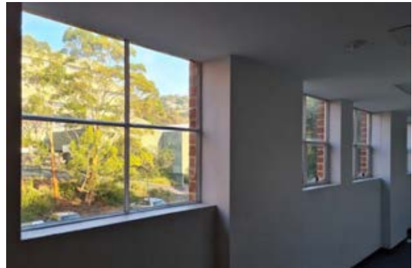
Building 40 – Hytten Hall Detail of an original steel window to the southern corridor of the original western wing Source: Paul Davies Pty Ltd
