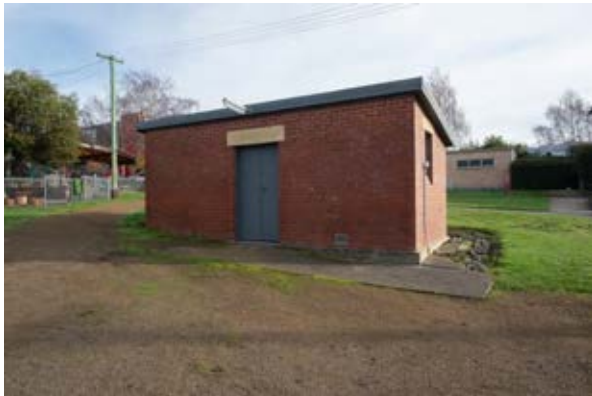
Building 53a – Brick Store Room Eastern elevation Source: Paul Davies Pty Ltd
