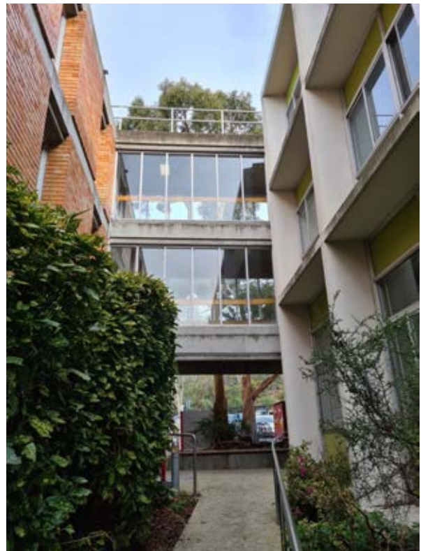
Building 29 – Humanities Building Glazed link between Humanities (image left) and Psychology (image right) – north elevation Source: Paul Davies Pty Ltd
