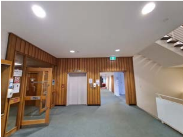
Building 13 – Physics Timber panelling to the main internal foyer Source: Paul Davies Pty Ltd
