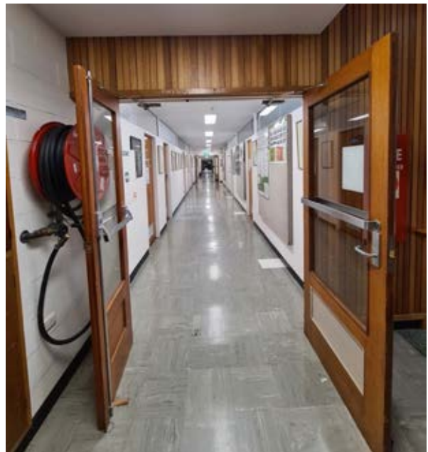
Building 34 – Life Sciences Building Typical central corridor of the original central wing with original timber joinery Source: Paul Davies Pty Ltd
