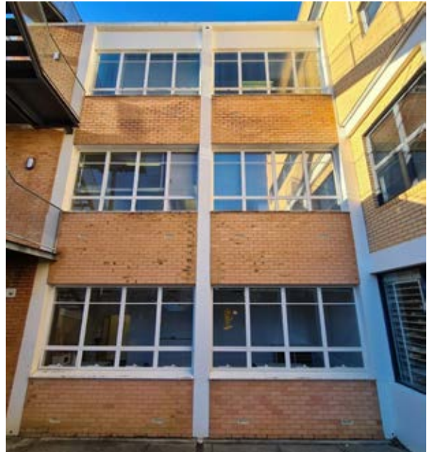
Building 12 – Geography, Geology and CODES 1969 southern extension – Detail of the western façade of the eastern wing Source: Paul Davies Pty Ltd
