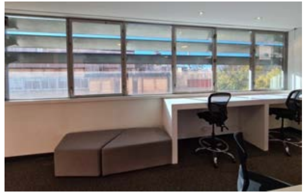
Building 23 – Library, Morris Miller Detail view of the aluminium glazed windows and external louvre blades for solar protection. Source: Paul Davies Pty Ltd
