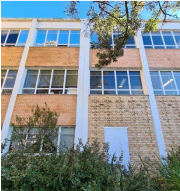
Building 12 – Geography, Geology and CODES Detail of where the 1969 southern extension occurs is evident with the double column and change in brickwork detail Source: Paul Davies Pty Ltd
