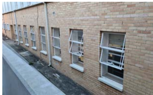
Building 8 – Engineering Building Southern façade – steel window detail Source: Paul Davies Pty Ltd
