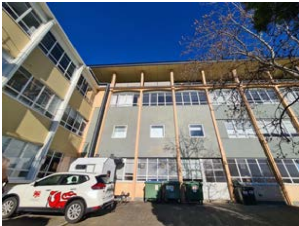
Building 12 – Geography, Geology and CODES Northern Façade facing Grosvenor Crescent Source: Paul Davies Pty Ltd
