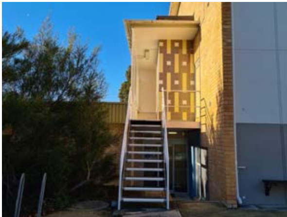
Building 8 – Engineering Building Tile detail on the northern-façade Source: Paul Davies Pty Ltd
