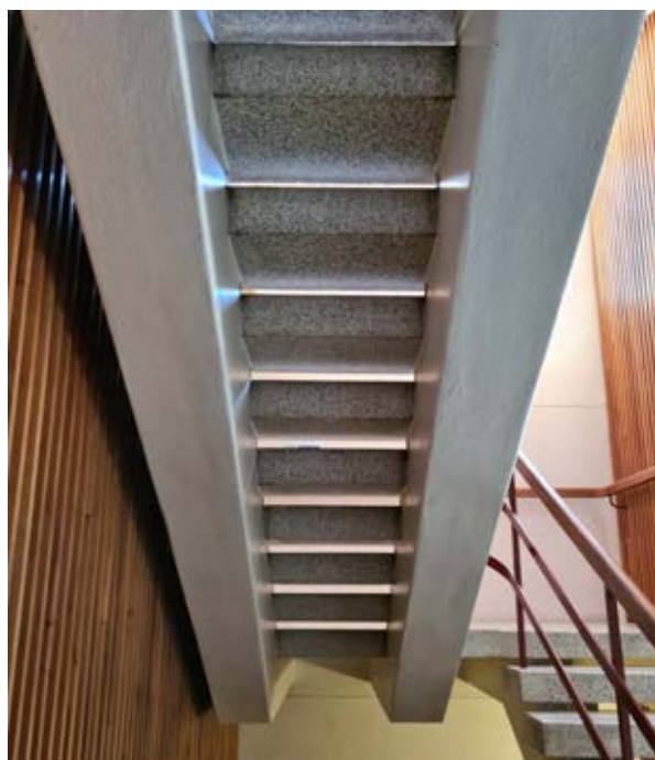
Building 26 – Psychology, Social Sciences Detail of the underside of the stair Source: Paul Davies Pty Ltd
