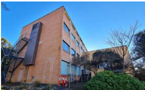
Building 13 – Physics Southern Wing, Southern Elevation showing the 1967 extension. Source: Paul Davies Pty Ltd
