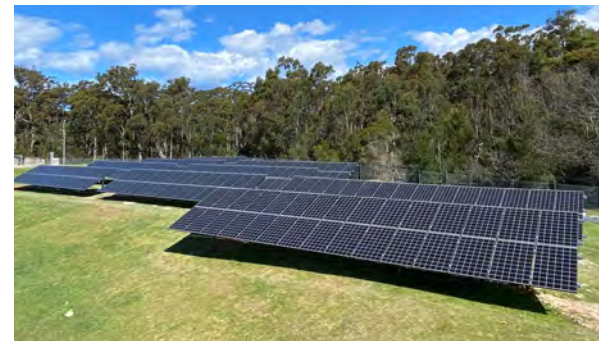
Figure 5: Shoalhaven’s Nowra waste treatment system PV panels https://www.shoalhaven.nsw.gov.au/files/content/public/for-residents/our-environment/sustainability/solar-array-vincentia.jpg?w=930&h=612
